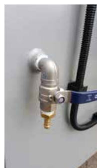
Low water cut out and manual water top up
