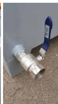
Quick drain tank with no blockage ball valve
