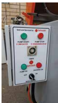
Steel electrical cabinet with IP65 electrics
